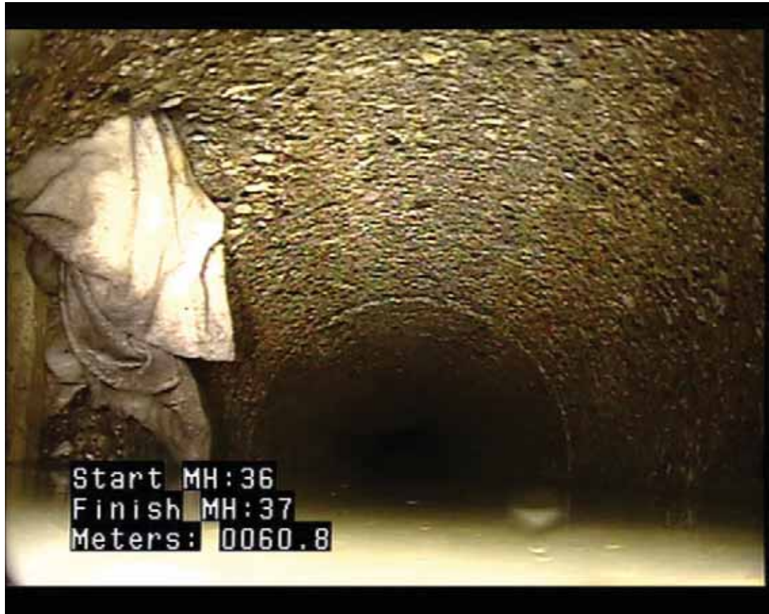
Photo 5.2: Ragged wrapped around service pipe along SP 125
