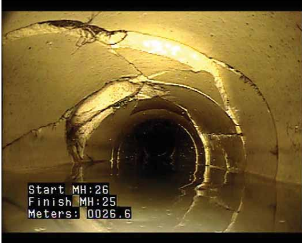
Photo 5.1: Severe Cracking and Fractures near service connection along SP 139
